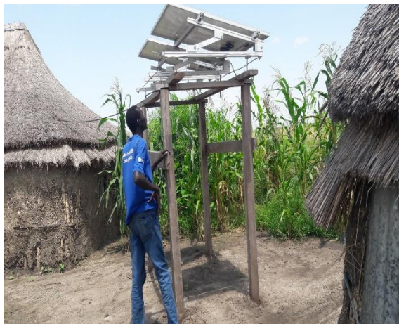
Figure 4: Ensuring access for vaccines in community hard to reach by installing cold chain in a locally constructed community building
